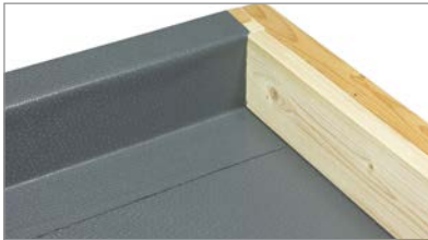
31. Complete the first parapet flashing so it finishes tight into the corner. Pre weld and final weld the flashing onto the roof surface.
