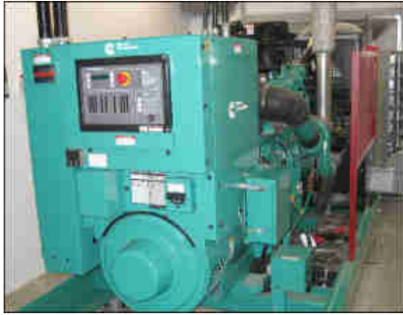
350KW Prime Power Diesel Generator
