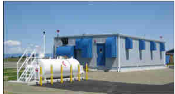
24' x 46' Building divided into Regulator Room, Generator Room and Workshop, c/w 350 KW Prime Power Rated Diesel Generator, 14 Switchgear Regulators, 10 Non-Regulated Cells and Novec-1230 Fire Suppression System.
