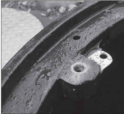
Internal view of pullpit with ground strap
