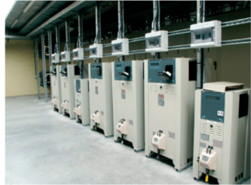
Fig. 2: MCR 3 in substation
