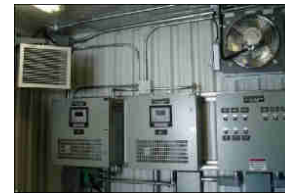
Fig. 2 Sentinel ALFEC with Liberty wall mounted CCRs, non-regulated panel, heating and ventilation.
