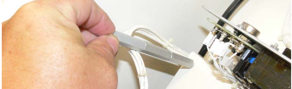
Figure 15: The three standoffs holding the relay support panel
