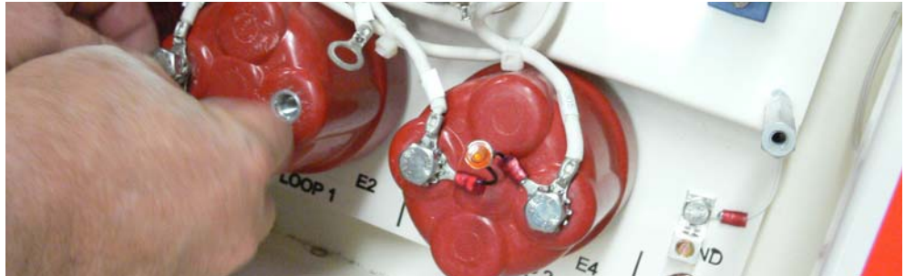
Figure 17: R1/R2, E1/E2 and E3/E4 wires shown
