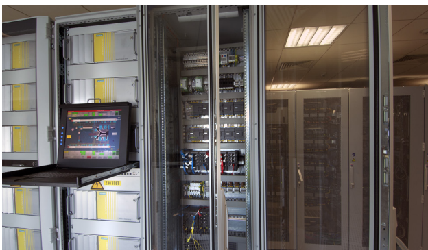
ALCS control room
