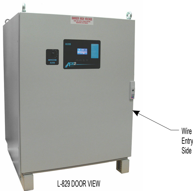
Figure 8: Wiring on Right Side of CCR
