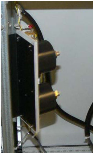
Figure 20: Output Lightning Arrestors
