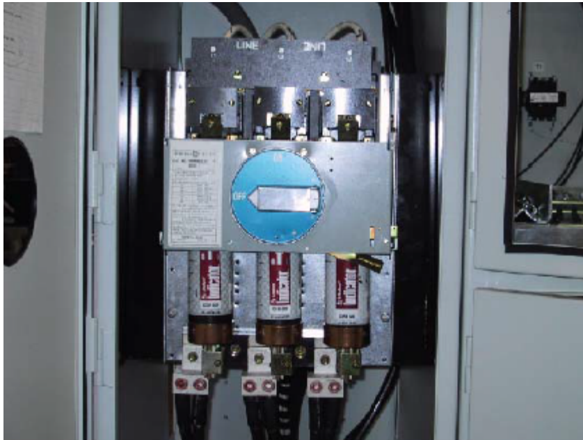
Figure 34: Incoming Power Bay with Door Open
