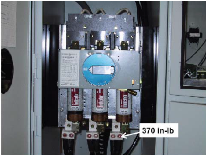
Figure 15: Fused Disconnect Switch
