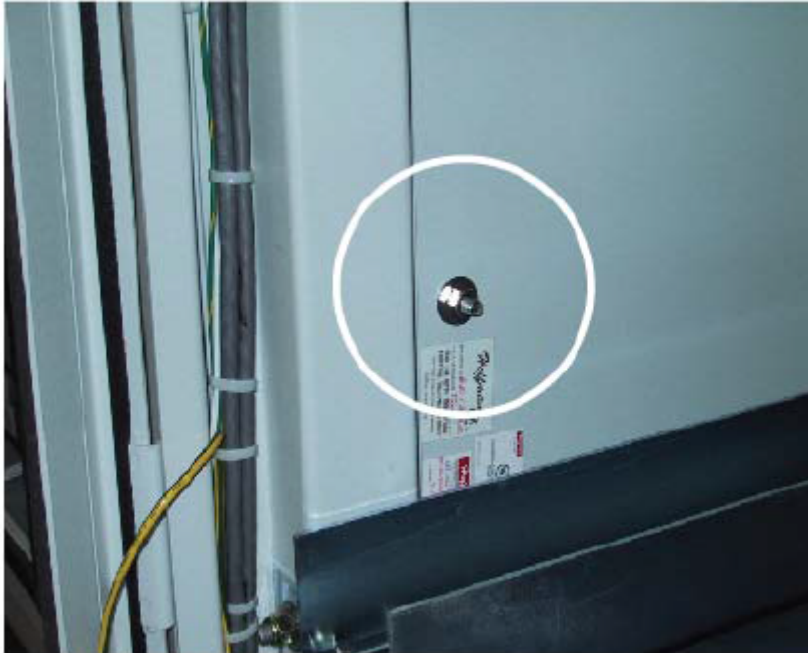
Figure 8: Inside of Cabinet Looking Left
