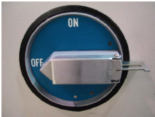
Figure 33: Disconnect Switch in OFF Position
