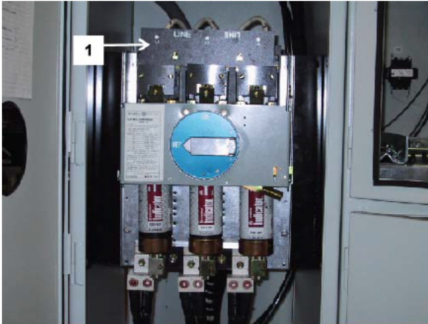
Figure 31: Fused Disconnect Main Power Connection
