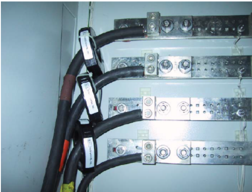
Figure 14: Current Transformer Installation
