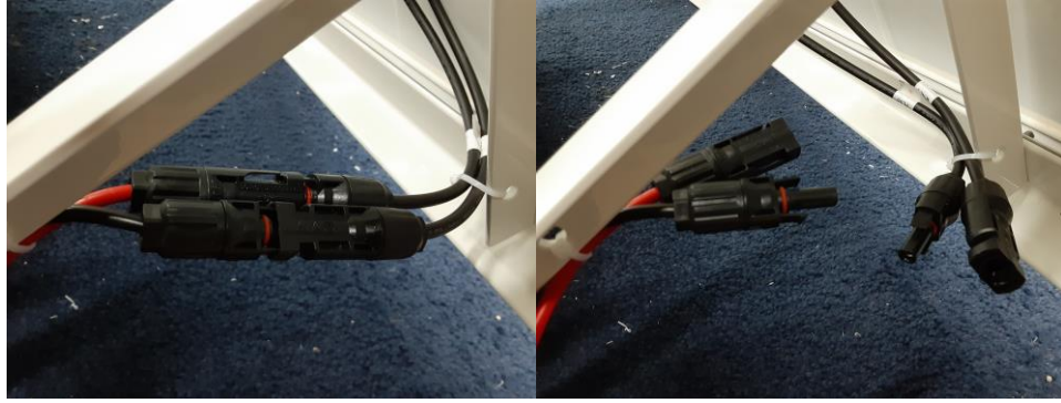
Figure 11. Solar Panel Connectors
