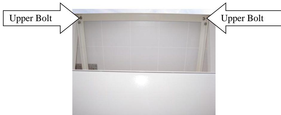
Figure 10. Upper Solar Panel Mounting Bolts
