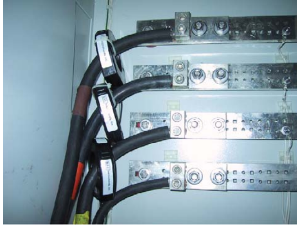
Figure 4: Current Transformer Installation
