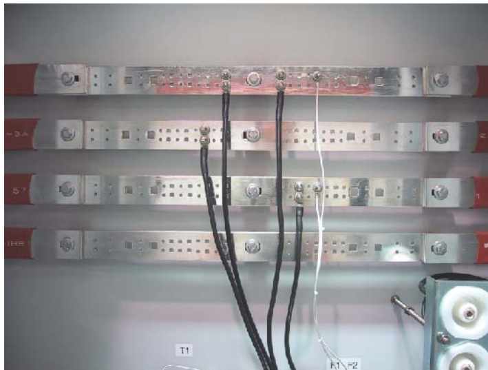
Figure 12: Powerpack Electrical Power Connections
