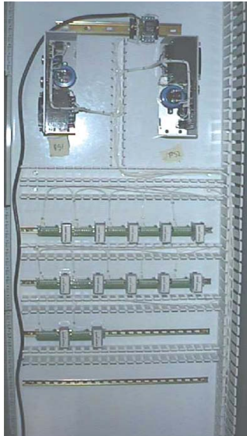
Figure 10: Typical Control Bay
